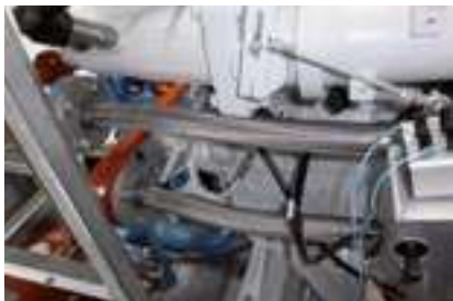
Stainless steel hose in a combined heat and power plant with swivel flanges
