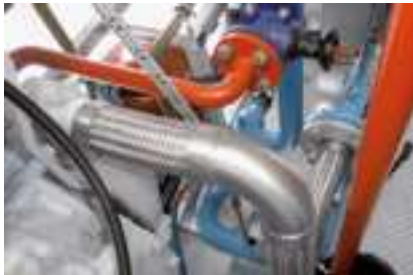
Stainless steel hose in a combined heat and power plant with 90° bend and swivel flanges
